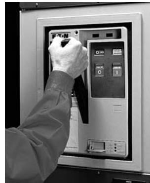
Through-the-Door Design for Human Interface with the Breaker Compartment Door Closed, for Example, Manually Charging the Stored Energy Springs
